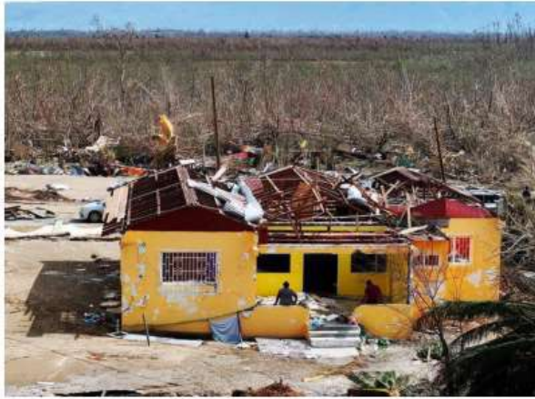
Roof gone: A house damaged by the hurricane in Crane Road, Black River, Jamaica, on Thursday. REUTERS
